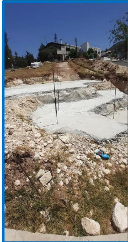
Ovalabout update, not much activity apart from concrete and pipes being laid.
